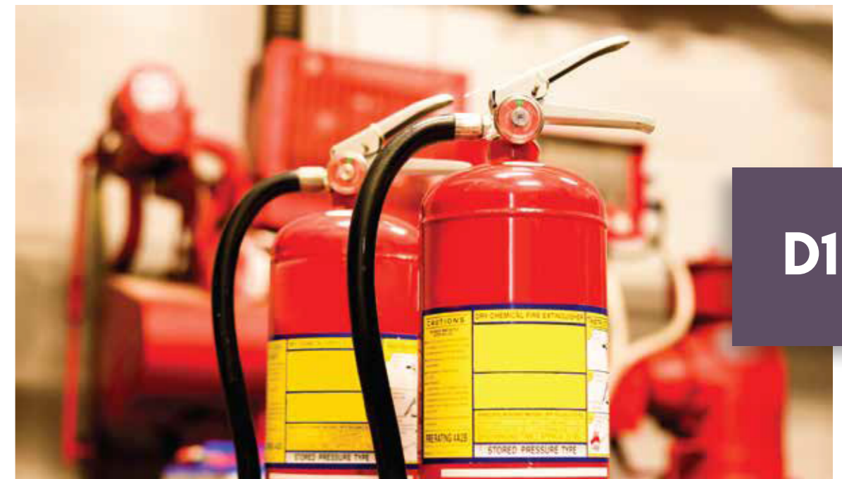
Fire fighting equipment including hose reel, wet riser, fire extinguishers and sprinkler system will be connected to the building management system
